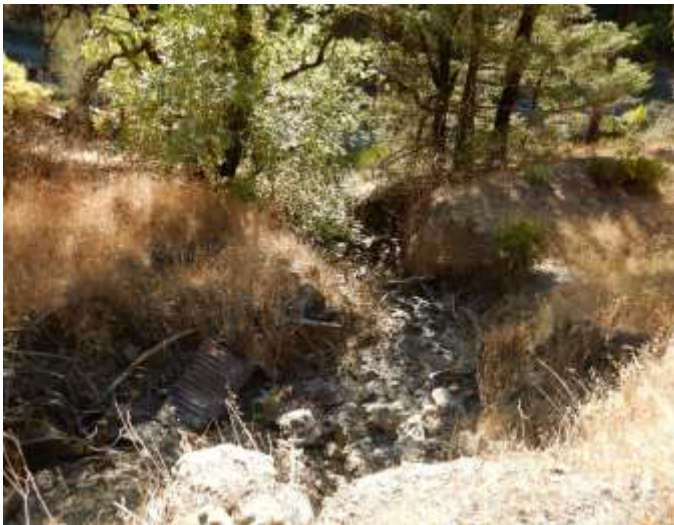
Figure 33. Eroding gully below road paralleling lower Tenmile Creek on Vassar property. 10/16/18.
