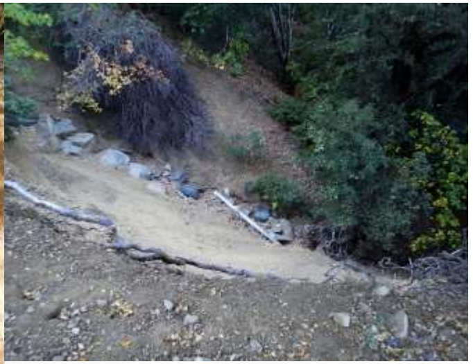
Figure 34. Road fill failure on upper Cahto Peak Road. 2/4/20.
