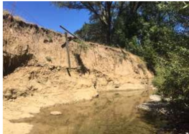
Figure 12 Bank failure on Streeter Creek dumping soil into prime fish habitat.
