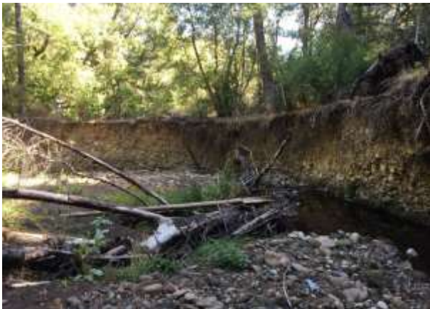
Figure 11 Mill Creek 300-foot-long failing bank on Feigon property.
