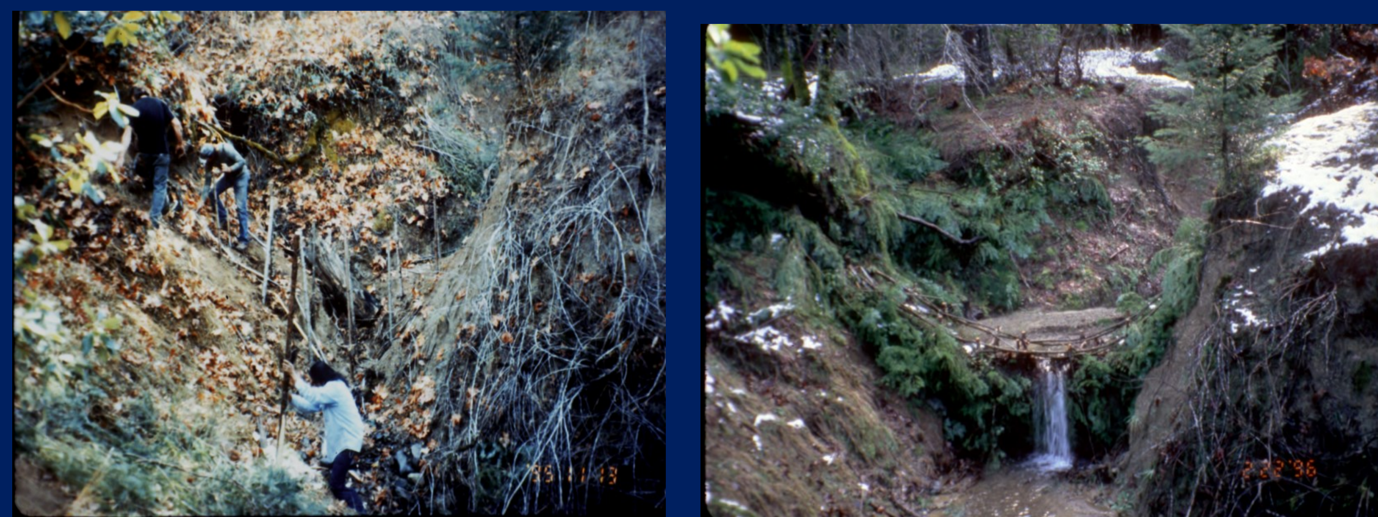
Gully erosion can cause siltation of streams, valuable agricultural soil loss and can drop the groundwater table making adjacent uplands less productive. BioEngineering Associates will be able to provide technical assistance free to Tenmile Creek land owners.
